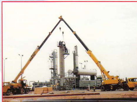
RISHA Gas Project - Jordan In Cooperation With AGRA MONENCO (AMEC) & PETRO-CANADA
