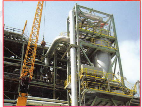
Arab Potash Expansion Falling Film Heat Exchanger at Hot Leach Plant
